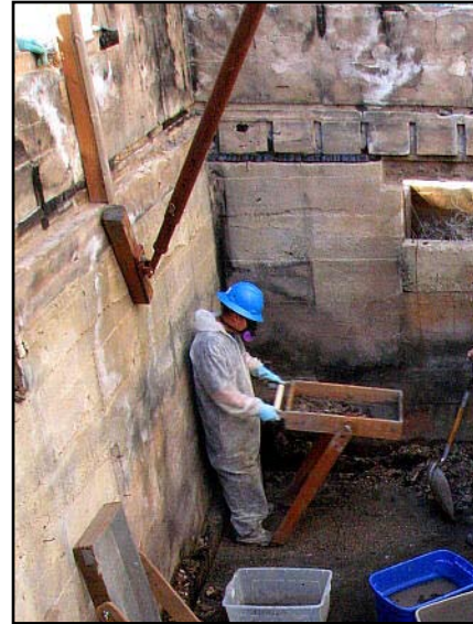
Haz-mat team in basement
